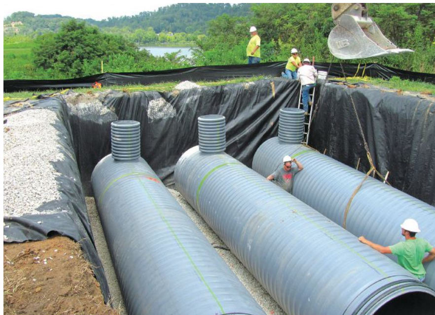
A Worthington, Ky., project sought to minimize sanitary sewer overflows into the Ohio River with 860 ft of 60-in.-diameter pipe installed in a three-row configuration.
